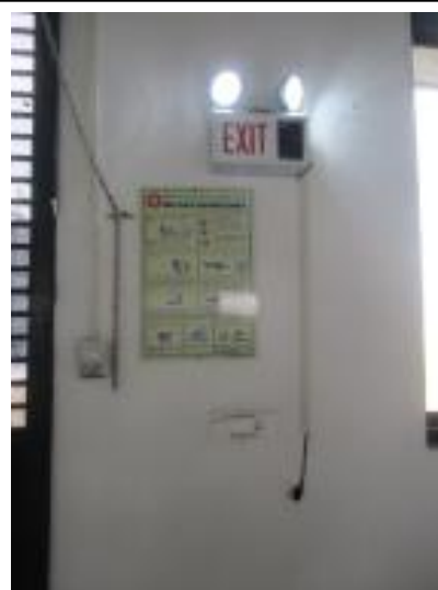
Emergency light backup.JPG
