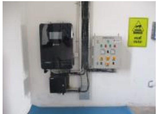
Electrical panel with mat.JPG
