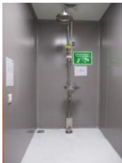
Eye wash station.JPG
