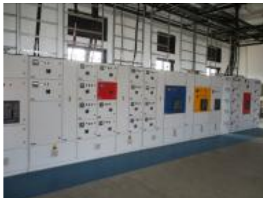
Electrical panel room.JPG
